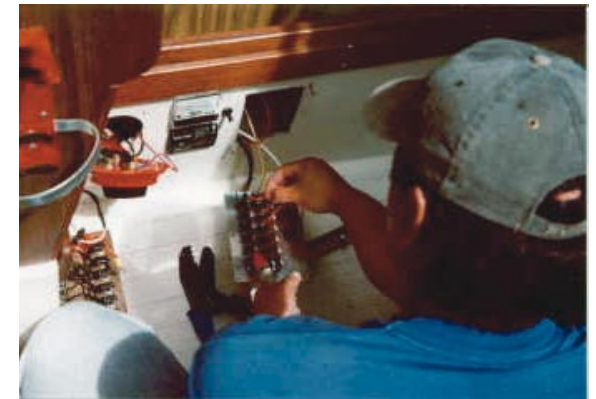
VESL student troubleshoots a boat's electrical system while working in a confined space.
