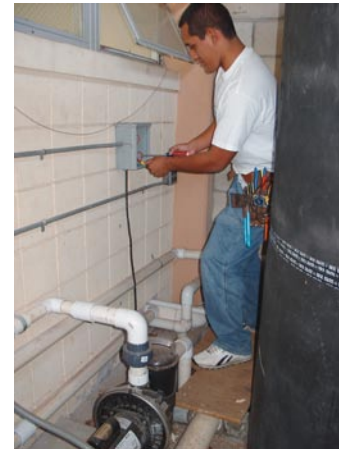
EIMT student works in a confined space on a slippery and uneven surface.
